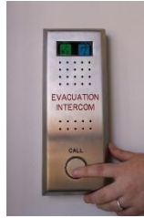
Figure 2: Example Evacuation Intercom located in Lift Carriage
