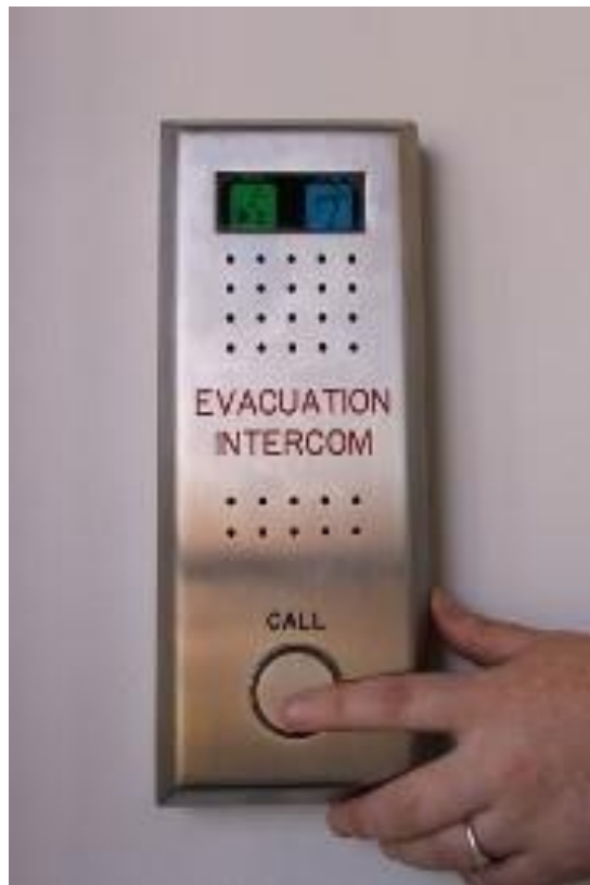
Figure 2: Example Evacuation Intercom located in Lift Carriage
